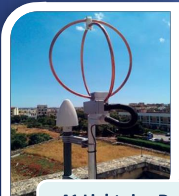
41 Lightning Detection and Tracking Systems
